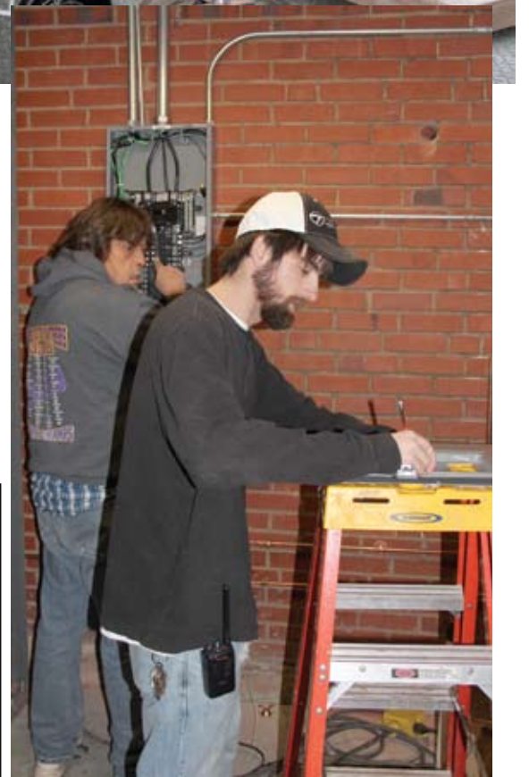
Paul Panning, left, and Kyle Staples, right- Continue work at the breaker box in the new Mound City weight room facility on Thursday, December 27. Maintenance director, Paul Panning, along with other custodial employees and ag students, has worked on every facet of the inside of the new space.
