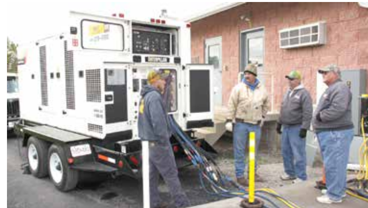
(From second left to right) John Dougherty, Kelly Graves and Randy Crowley - Chat with a Caterpillar Inc. representative, far left, on Wednesday, Oct. 23, while running electrical tests for a new generator for the water plant in Mound City, MO.
