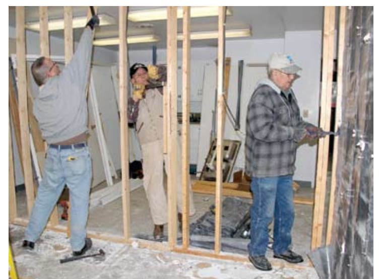
Paul P. Shutts American Legion Post #121 members- Began working on the huge project of making their new space usable from the cut up space of a portion of the old clinic in Mound City on Monday, February 20. Pictured left to right, taking out the old x-ray room with its lead lined walls are Randy Miller, Maurice Smith and J.M. Jackson.
