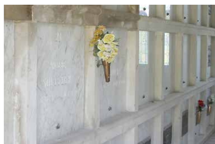
The vaults in the Mound City Mausoleum - Have remained fairly unscathed from the extreme deterioration of the structure's roof over of the years. Granite and marble are very durable with minimum maintenance if the roof keeps out the elements.
