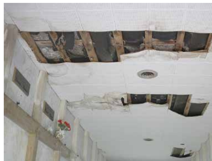
Much of the ceiling in the Mound City Mausoleum - Has fallen onto the tiled floors below due to a deteriorated roof, left unattended for years, that has allowed rainwater to damage the ceiling. The marble plates at each burial chamber are unharmed.
