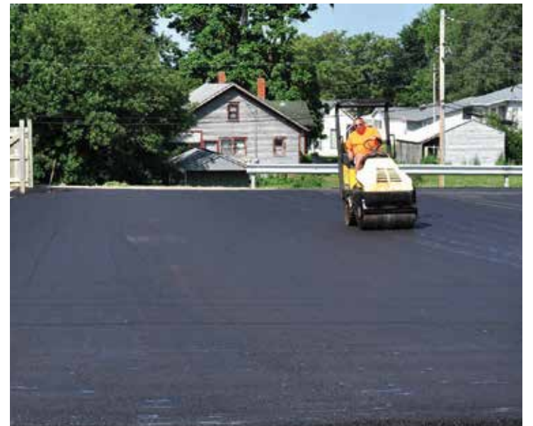
The parking lot east of Mound City R-2- Was asphalted on Tuesday, July 16, in Mound City.
