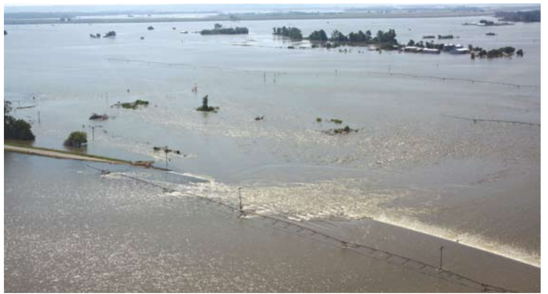
What appears to be an even more destructive current- Than that of the flood of 2010, rushes over Highway 111, just west of the junction of Highway 111 and Highway 118, at the north end of Big Lake. MoDOT has the financial burden of highways like this that are being washed away. The floodwaters have receded very little, but the extent of the destruction for the county itself has already been estimated to exceed $7,000,000 in infrastructure damage - which includes county roads, levees, bridges, and culverts.
