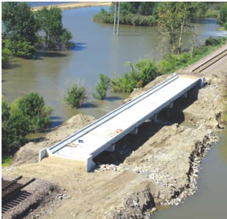
One of the six railroad bridges- Being constructed along the approximately 3.5 miles of railroad track between the Missouri River at Rulo, NE, and the town of Fortescue, MO, appears to be nearing completion. The new bridge appears to be at the current track height, and a slough has already been dug beneath the bridge to allow for draining of floodwater from the north side of the tracks to the south side and theoretically back to the Mighty MO.
