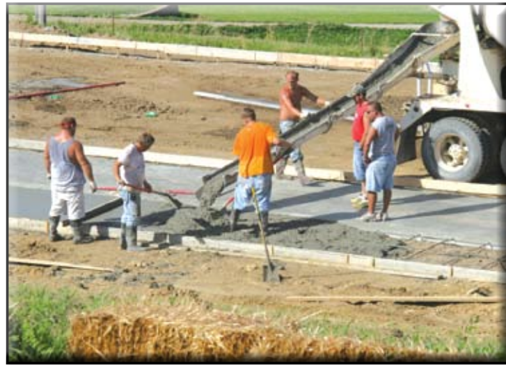
Pictured above is concrete being poured by Jeff Karsten's concrete crew- Last week. The new press building sits north of Mound City at the junction of Highway 59 and Highway N. The workers were able to get the pad for the building finished amidst the sweltering heat.
