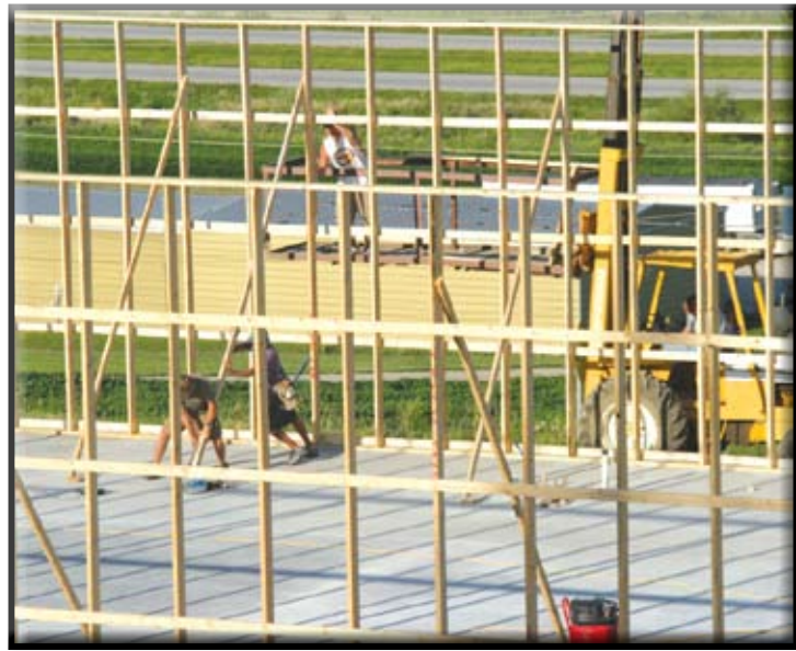
Walls started going up- Immediately after the concrete crew was finished. The Matt Phillips Construction crew is shown working on Tuesday, August 3.
