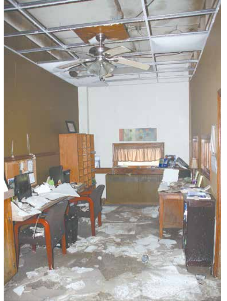
Fallen ceiling tiles and water damage - Cover the floor and desks of the counselor's office at Nodaway-Holt R-7 on Wednesday, Sept. 10, hours after a storm swept through on Tuesday night.
