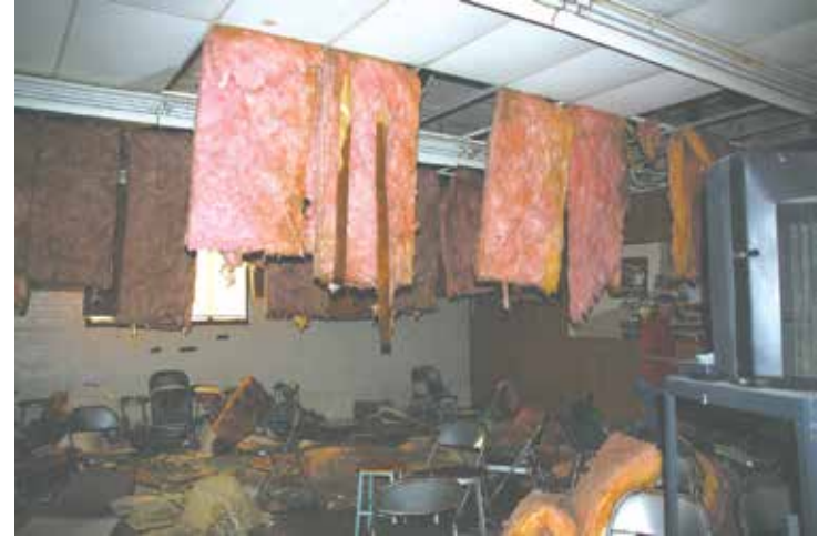
The damaged Nodaway-Holt R-7 band room - Is shown here. According to Superintendent Karma Coleman, the band room and the vocational agriculture building were "a total loss." Repairs are expected to take anywhere from four to six months.
