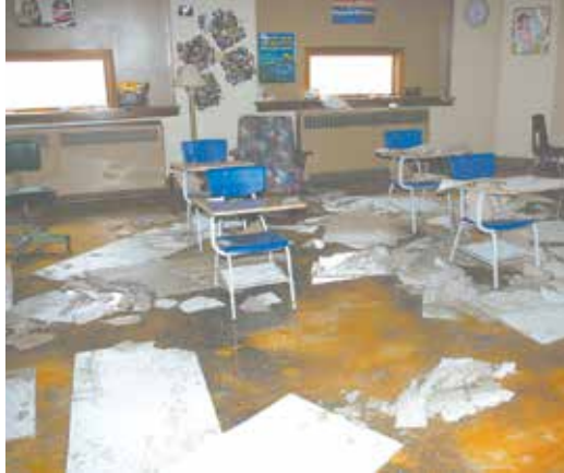
Crumbled ceiling tiles and water - Litter the floor of a classroom at Nodaway-Holt R-7 in Graham, Mo., after a severe storm ripped through the area on Tuesday, Sept. 9.
