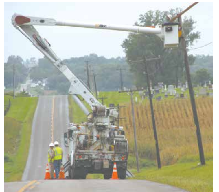
Kansas City Power and Light crews - Work to restore power after the Tuesday, Sept. 9, storm caused 1,655 customers to lose electricity.
